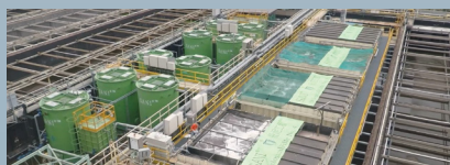
SANI launched a full-scale trial at Hong Kong's Shatin Sewage Treatment Works in the summer of 2014.
